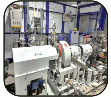
Engine testing Facility
